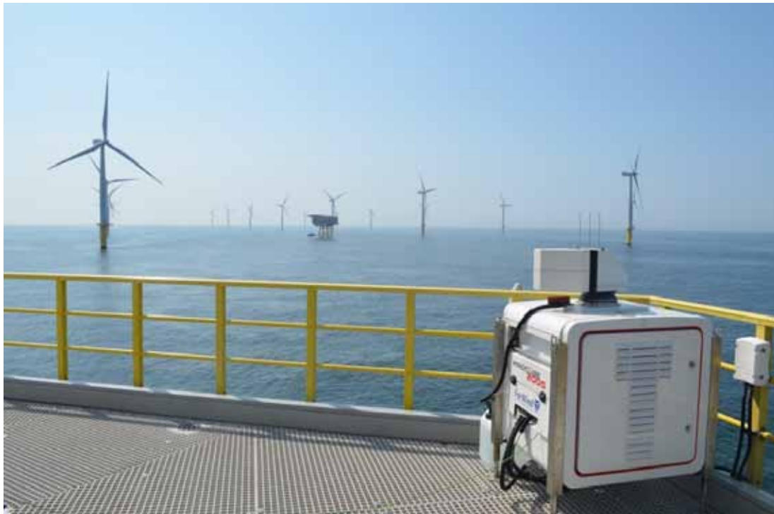
Figure 1: Lidar system with large measuring range on the transition piece of a wind turbine in the Riffgat offshore wind farm
