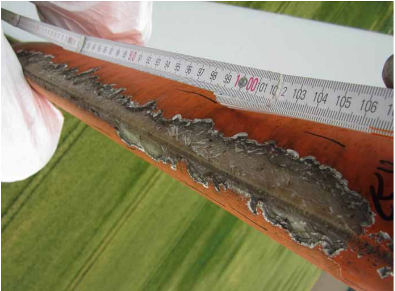
Figure 1: Damage to wind turbines such as this one at the leading edge of a rotor blade requires extensive servicing and the use of special forces suitable for high altitudes. (Source: MB Bladeservice Einbeck)
