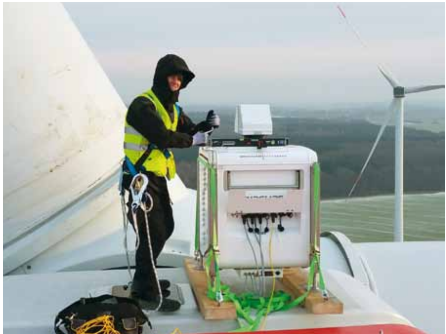
Figure 2: Installation of a long-range Lidar measurement system on nacelle of eno 114 wind turbine
